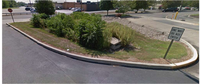
BIORETENTION BASIN NOT MAINTAINED
